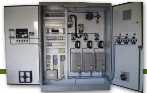
Triplex Pump Control Panel
